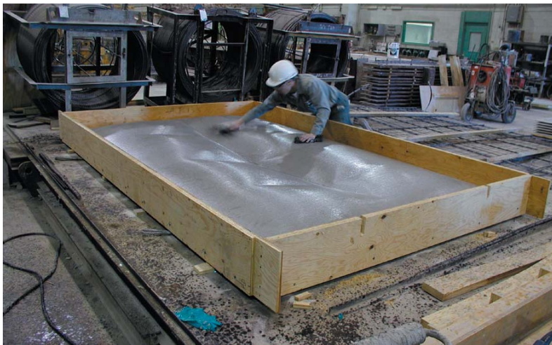
Figure 8. A “direct-cast” concrete panel being prepared as a mold for the “inverted cast” shell panel shown in Fig 9. The concrete of the mold panel is sealed and then coated with release oil prior to casting.
