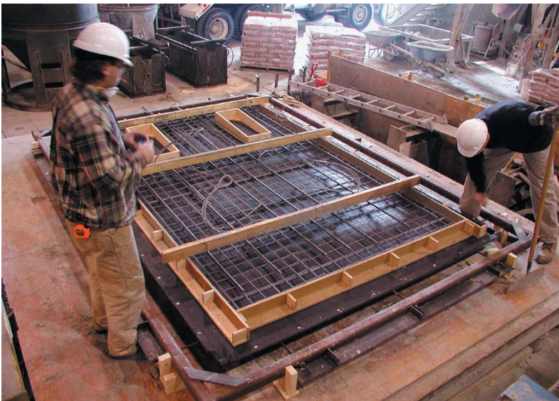
Figure 3 (below). Complete formwork prior to placement of concrete: The fabric formwork membrane has been pre-tensioned over the lower frame and intermediate supports, and the upper frame and reinforcing is in place above the fabric membrane.
