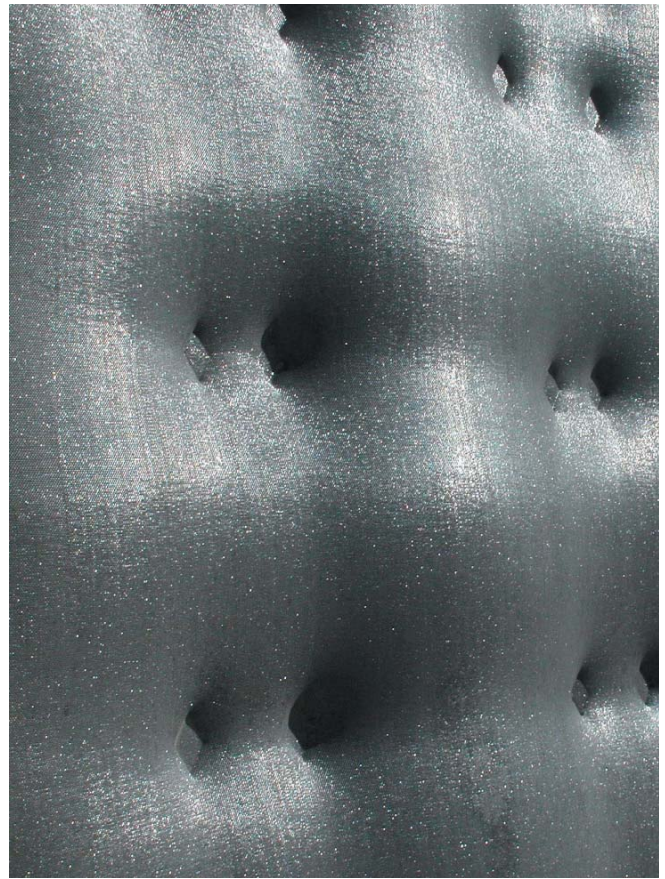
Figure 4b. Close-up view of the surface texture of the "direct-cast" panel shown in Fig. 4a. The permeable geotextile fabric formwork gives a sensual and immaculate finish.
