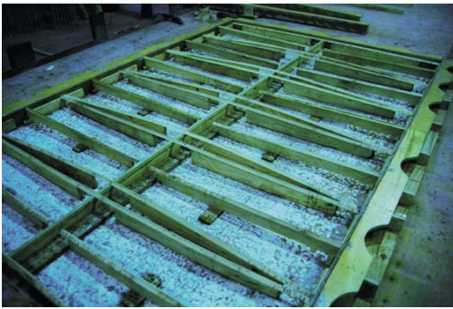
Figure 10. Lower frame and intermediate supports used to produce the Figure 11 "direct-cast" panel, which in turn produced the Figure 12 GFRC shell panel.
