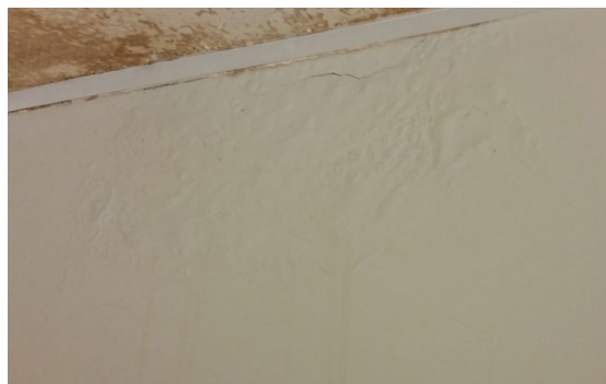
Figure 5. Peeling, sagging or bubbling paint on surfaces.
