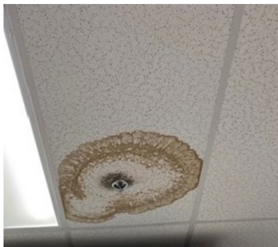
Figure 4. Staining and discolouration on ceiling tiles
