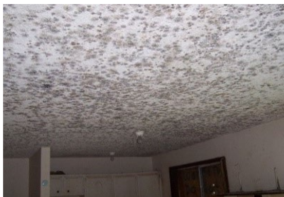
Figure 3. Large mould area, a single patch is larger than 3 m 2
