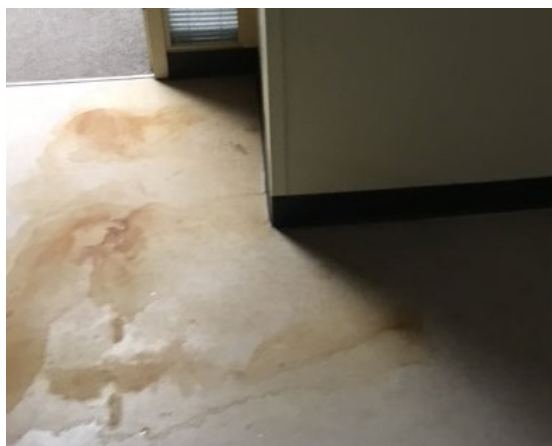
Figure 6. Staining and residue from water accumulation or condensation.
