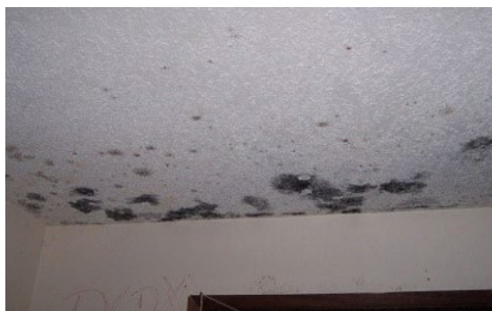
Figure 2. Medium mould area, more than 3 patches or an area greater than 1 m 2 but less than 3 m 2
