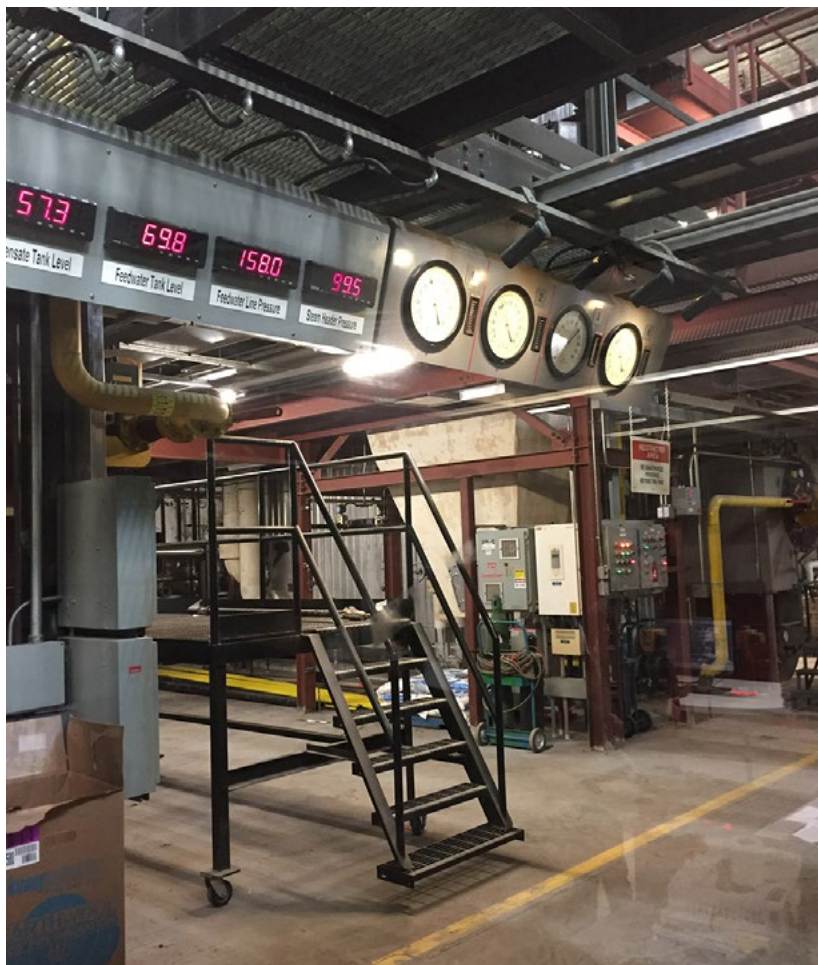
Boiler Room at the University of Manitoba Central Energy Plant
