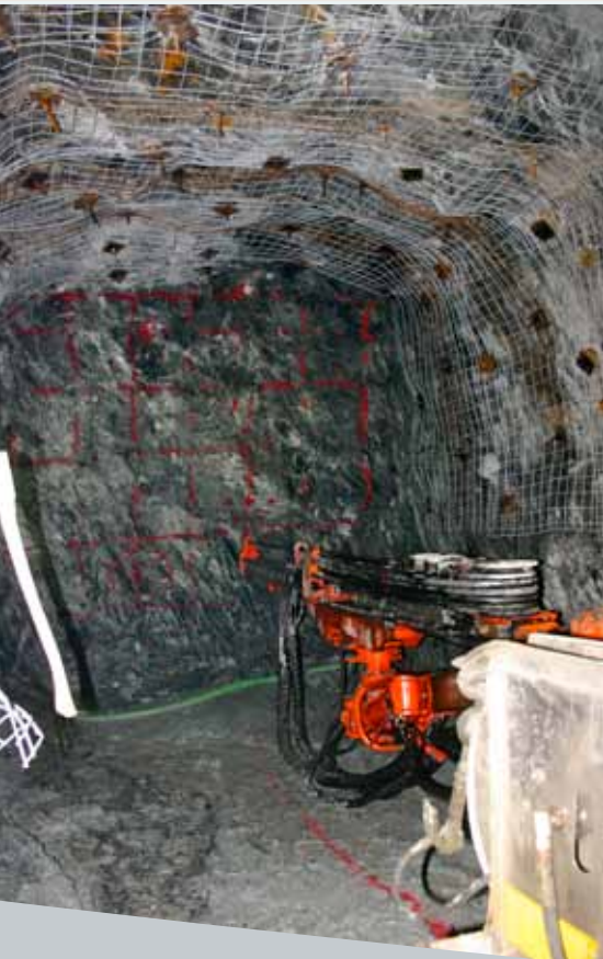
Pictured left, an active face on the 33 level, Red Lake Mines, Goldcorp. Drilling was stopped so that students could examine the face and discuss the drilling technique. The image also shows the ground support (i.e., rock bolts and screening) necessary to support the walls and back (ceiling) of the drift (tunnel). Photo Credit: Jeff Young.
