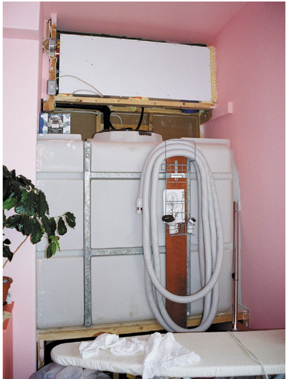
The rainwater storage tank and system on the second floor of the WBDC Healthy House was created and built by Burton Boryen from Advanced Design Build Inc. (Photo: Jessica Roder)
