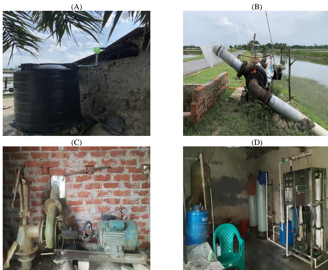
Figure 3.4 Technologies being used for water supply: (A) Rainwater harvesting (RWH) (B) Low-lifting pump (LLP) (C) Deep submersible pump (DSP) attached with deep tube well (DTW) (D) Reverse osmosis plant (RO).
