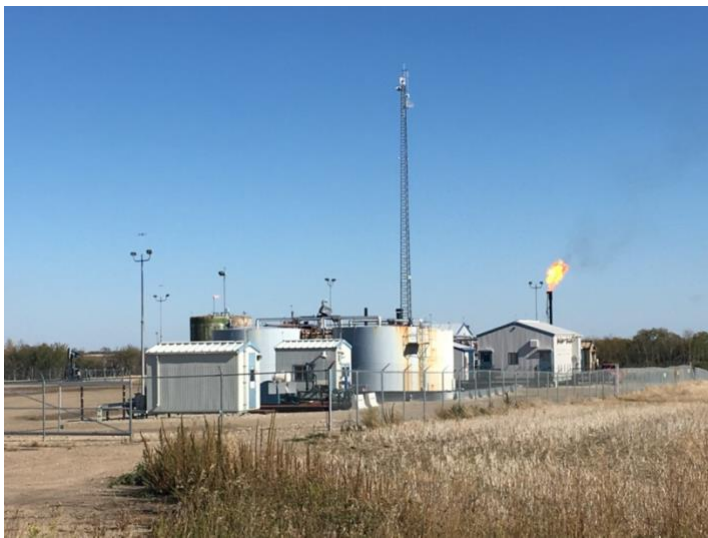
Figure 14: Battery Site with Flare Stack (ex. 2), Manitoba
