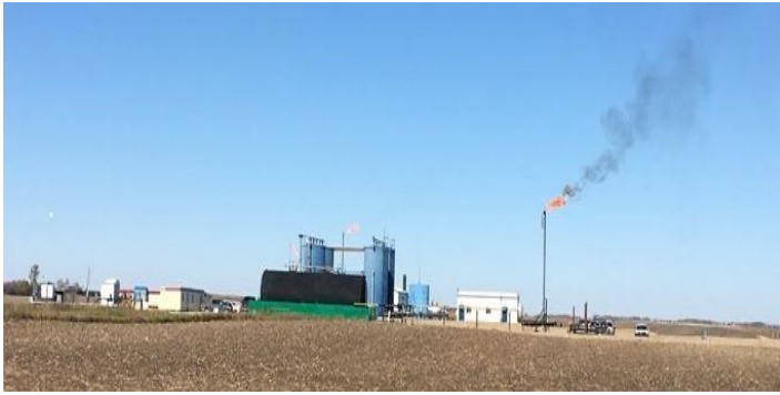
Figure 15: Battery Site with Flare Stack, Manitoba
