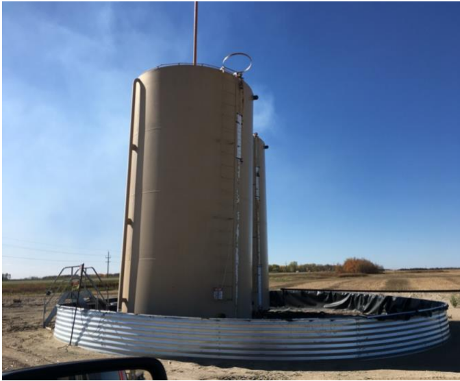
Figure 11: Storage Tank, Manitoba
