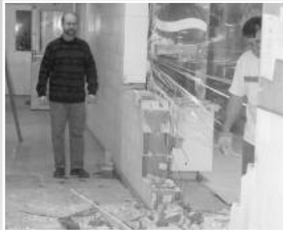
Residence Kitchen DURING Renovation with Dean of Residence Paul Lampman looking on.
