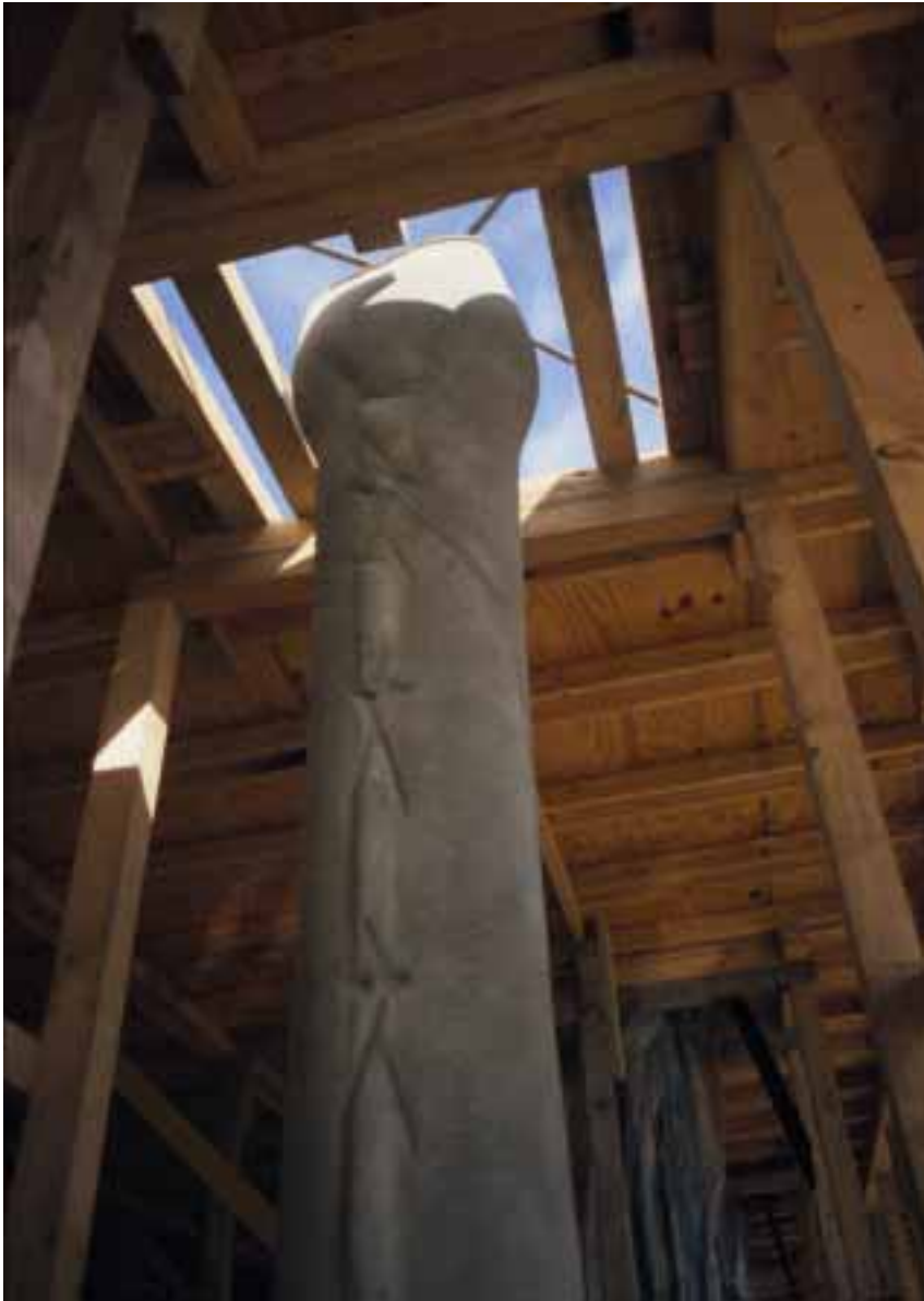
Fig. 3. Typical concrete column cast from fabric formwork shown in fig. 1. Architectural design and detailing are the result of natural deflections in the formwork fabrics caused by the hydrostatic pressure of the wet concrete.
