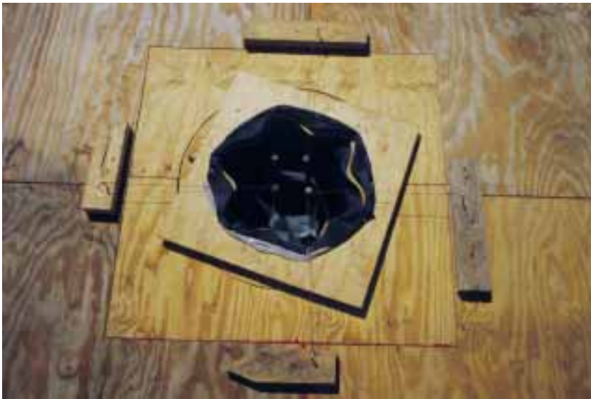
Fig. 9. View of a column fabric formwork meeting the top of the roof slab formwork deck. The (dark blue) stretch knit liner is seen attached to the center of a plywood ring that is free to rotate in the roof formwork deck.
