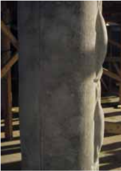
Fig. 7. Concrete column shaft showing finish free of bug holes, but with slightly 'blotchy' appearance due to uneven nature of concrete mix.
