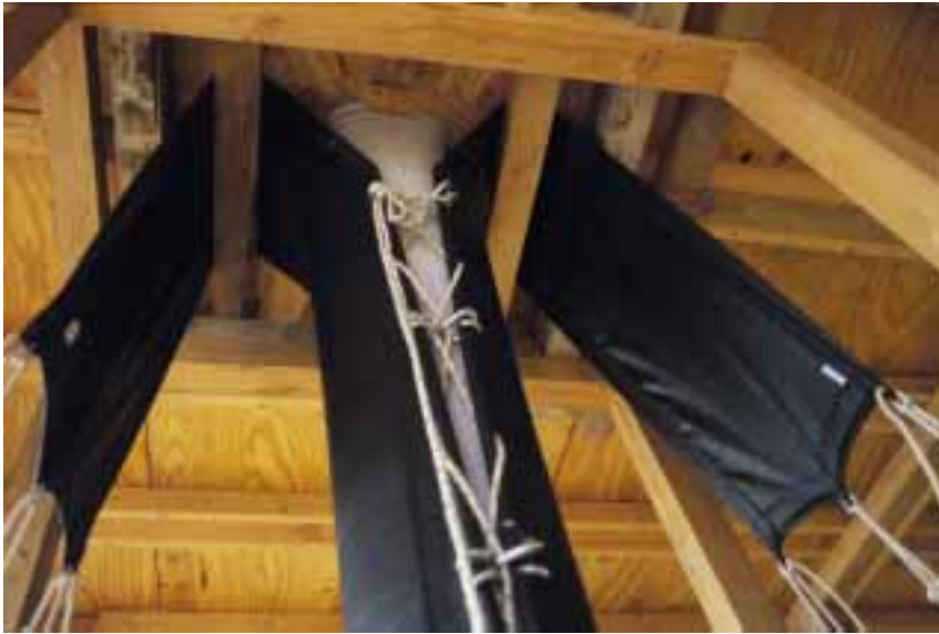
Fig. 6. Fabric Formwork fully installed and awaiting concrete placement. Note how the (black) outer jacket is rove over its 4x4 “sheaves” for vertical pre-tensioning. Also note how the (white) stretch-knit liner meets the underside of the roof slab formwork, adapting to in its own specially cut profile.
