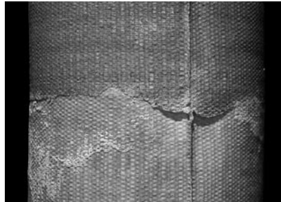
Column 'back' showing the typical overlapping 'bump' of cement paste at the joint between wood blocks.
