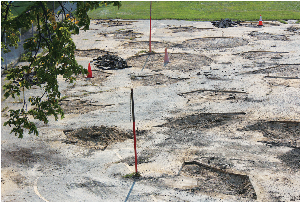
图06 挖掘：现场挖出的所有材料都留在场地内。 Fig.06 Excavating: Every bit of the excavated materials remained on site.
